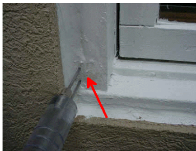
Rotted wood needs to be replaced.
