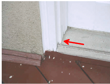
Suggest sealing door thresholds.
