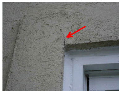
Cracking may be a result of the underlying damage.
