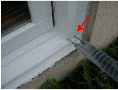
Replace all rotted wood.
