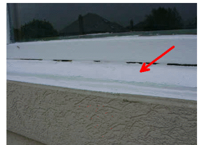
Rotted window sills need to be replaced.
