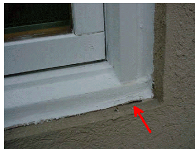
Perimeter sealants have aged and need replacing.
