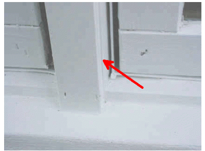
Window mullion joints need to be sealed.
