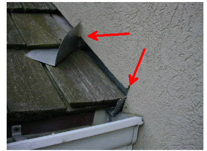
Improper kickout flashings. Replace all to current std.
