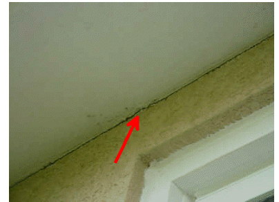
Gaps at the soffit should be sealed.
