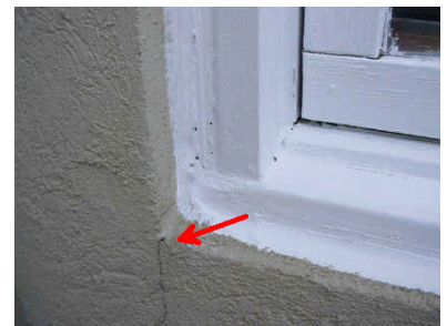
Cracking may be a result of the underlying damage.
