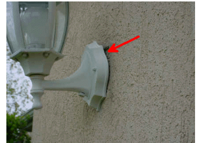
Light fixtures need to be secured and properly sealed.
