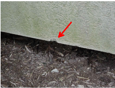
Repair typical mower damage.
