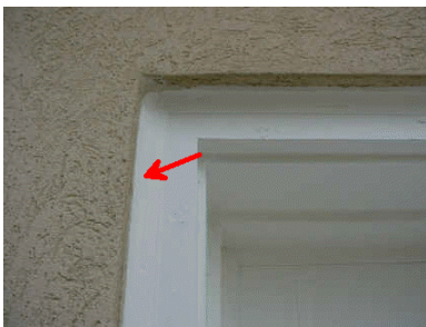
Paint hides aged sealants. Time to replace all perimeter sealants.
