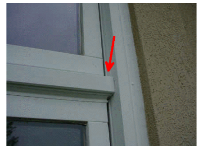
All wood window construction joints need to be sealed.
