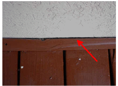
The deck diverter flashing needs to be resealed.
