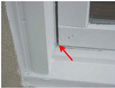
Window miter joints need to be sealed.
