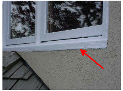
Inadequate perimeter sealants replace all.
