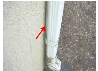
Gutter is damaged from winter freeze. Repair and seal.
