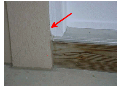
Replace all aged sealants
