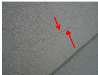
Repair compression cracking at entrance.
