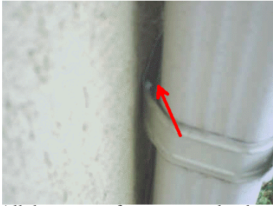
All downspout fasteners need to be sealed.
