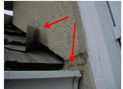
Improper and missing kickout flashing. Replace all.
